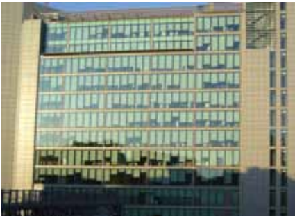
Over-glazed facades not only lead to unnecessary heat loss in winter and demand for air conditioning in summer, but the excessive glare means that occupants will close blinds increasing the demand for artificial lighting.
