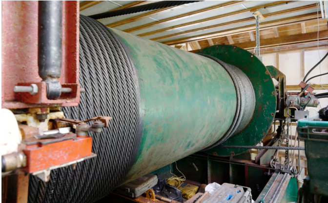
The steel cable that connects the two railway cars on the CAT cliff railway.
