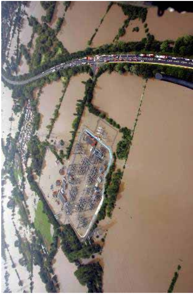
Walham substation, Gloucestershire, courtesy Geodesign Barriers Ltd
