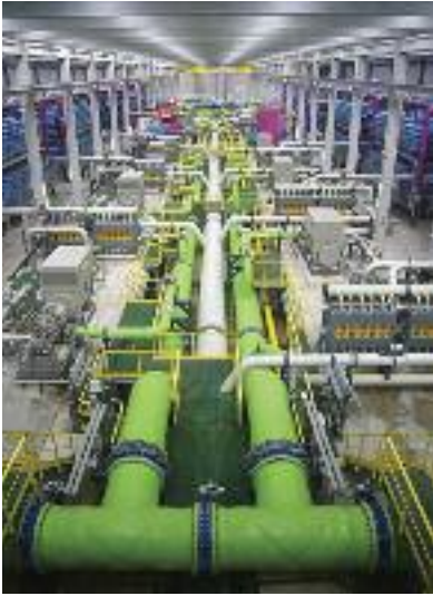
Figure 3: Desalination Plant, Llobregat, Spain
