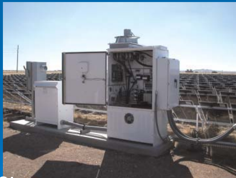
Xantrex PV150 system inverter Tucson Electric Power Company
