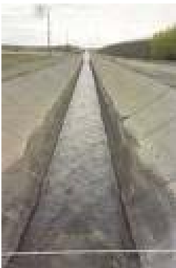
Figure 1: Open channel drainage system
